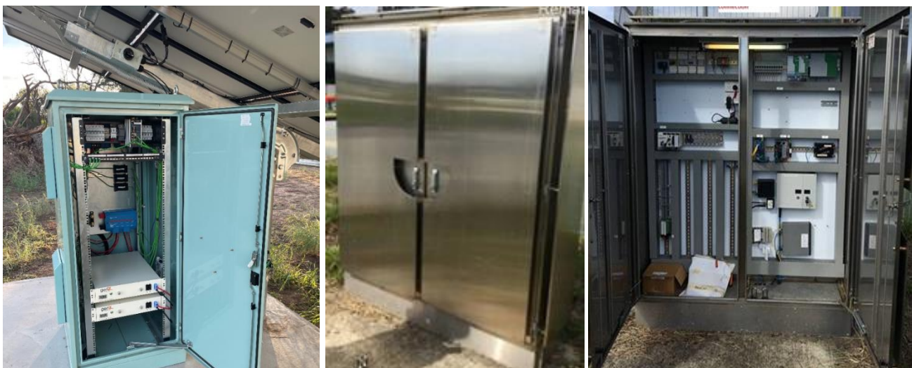
Figure 7. Examples of External Rack mount and wall mount customer supplied telecoms cabinet/enclosure
